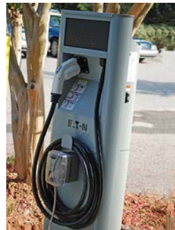
EV Charging Station
